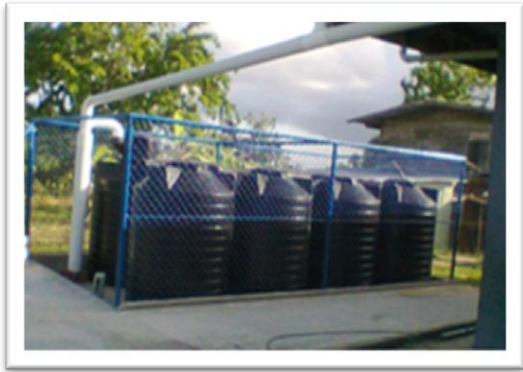
Rainwater Harvesting at Invernes
